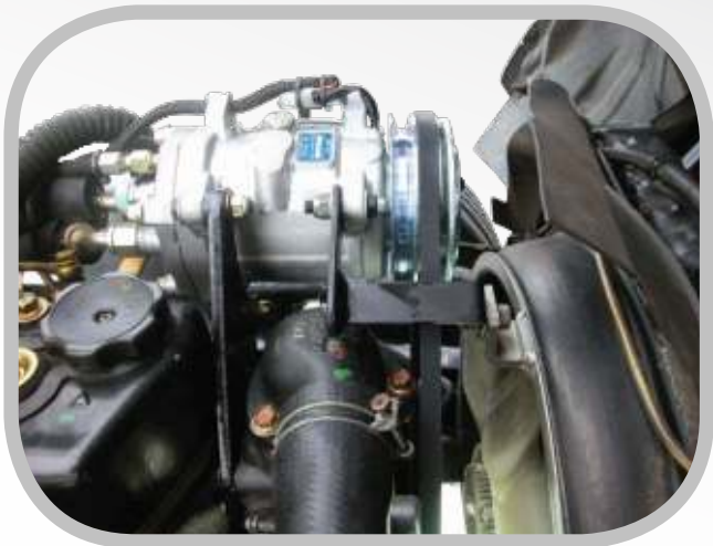
Compressor mounted to engine.
